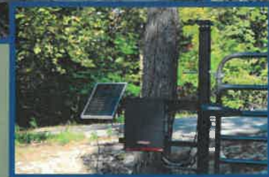
New solar-powered security gate at the Porto Cima storage facility
